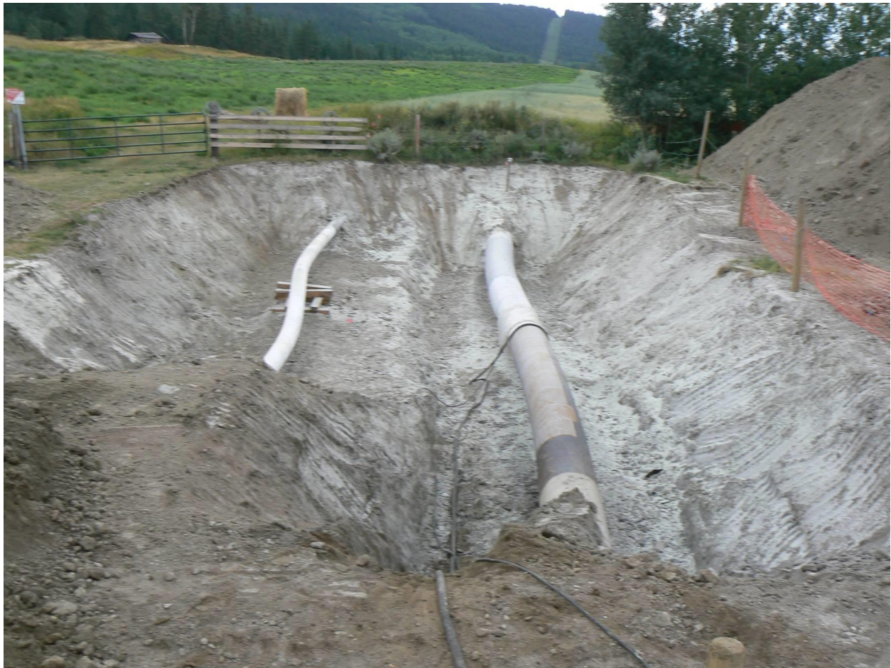
Figure 8-73 Looking south at the south flank of a deep-seated active translational landslide. A 12-inch oil line is located on the left and a 30-in natural gas pipeline is located on the right. The section of pipeline in the upper portion of the photo is located in stable ground with the section of the pipeline at the bottom of the photo being dragged downslope by approximately 1 in (25 mm) of annual movement. (Photo by: D. Dewar, Year: 2008)
