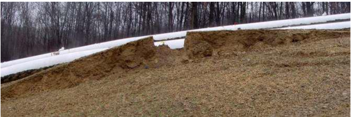
Figure 1-8 A segment of a pipeline that heaved out of the ground
