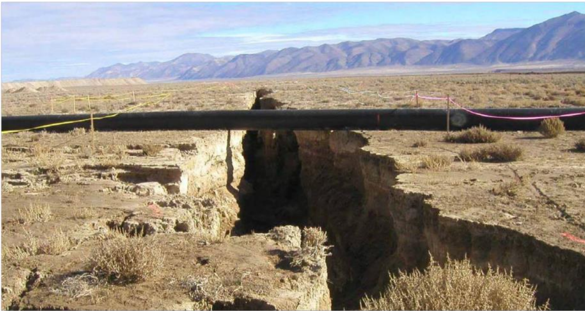
Figure 2-39 Earth fissure in Nevada at a mine facility with an above-ground mine process pipeline (Source: AMEC presented in 2004 ADOT workshop [83])
