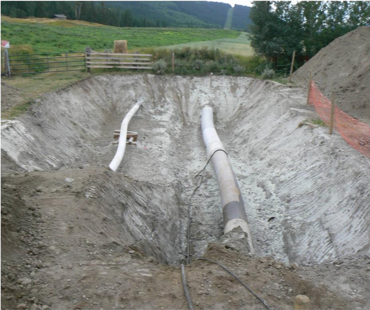
Figure 2-32 Pipeline bending associated with transverse downslope movement of large deep-seated, very slow moving translational earth slide. Both a 12-inch and 30-inch pipeline are bent by approximately 6.5 ft of landslide movement over the past 50 years. The fixed (stable) end is near the top of the photograph with movement from left to right. (Photo by: D. Dewar, Location: Central British Columbia, Year: 1998)
