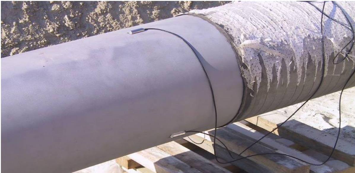
Figure 8-82 Three position strain gauge install on 36-inch natural gas mainline ready for recoat and backfill (Photo by: D. Dewar, Year: 2008)
