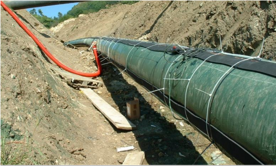
Figure 8-88 FO Cable monitoring install with three strain/temperature tapes oriented at roughly 12, 4, and 8 o'clock along a 500-meter length of pipeline in a landslide. (Photo by: Smartec, Year: 2003)
