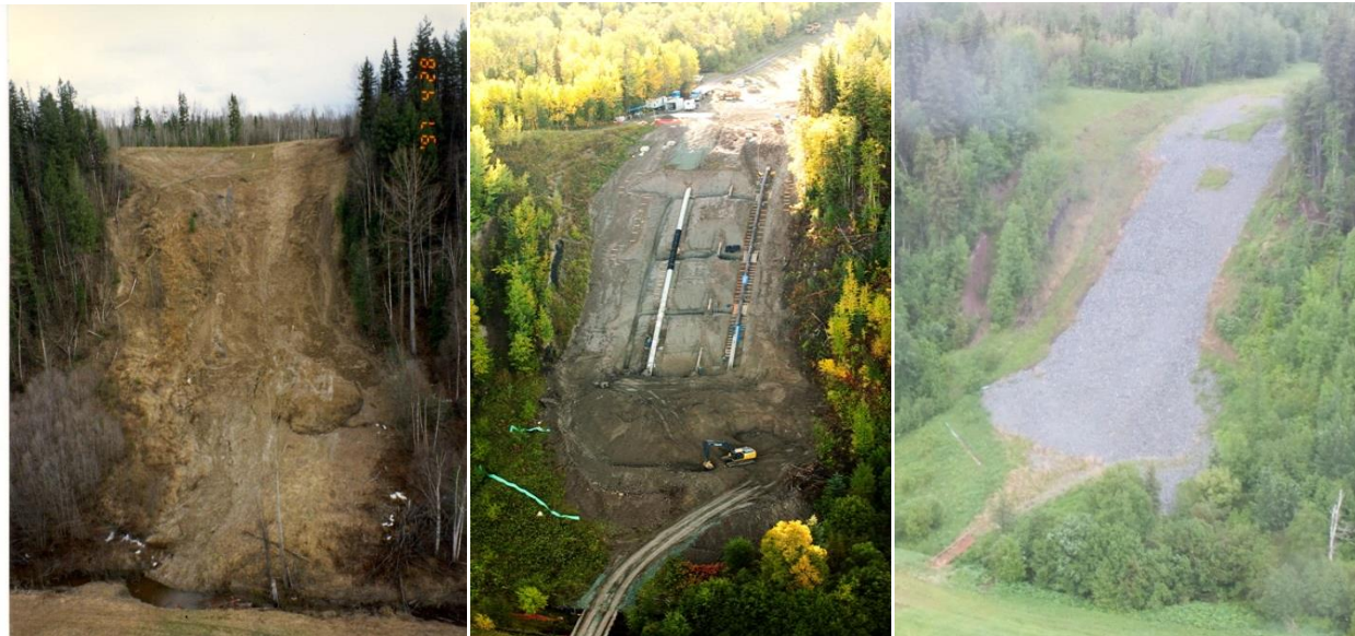
Figure 8-14 Stabilization of shallow earthflows in glaciolacustrine soils on pipeline ROW by removing all softened material (primarily pipeline backfill), installing a network of French drains and covering the pipeline by installing a blanket (upper slope) and buttress (lower slope) or riprap material. (Photos by D. Dewar, Location: Central British Columbia, Year: 1997, 2008, and 2012, respectively)
