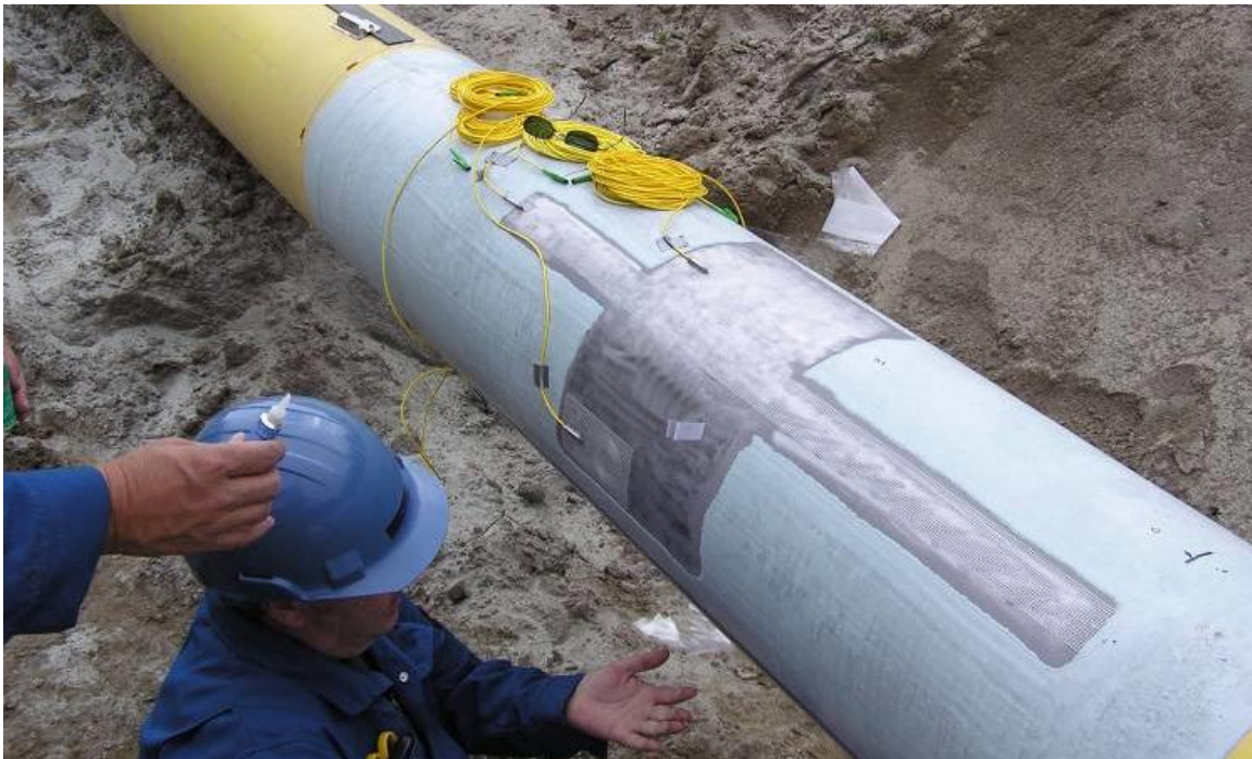
Figure 8-86 FO strain gauge installation with longitudinal and axial gauges (Photo by: E.C. McClarty, Year: 2005)
