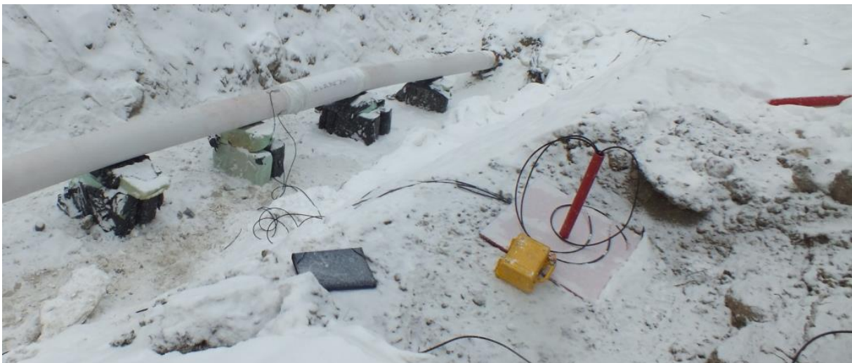
Figure 8-83 Four position strain gauge install on a 12-inch oil line ready for recoat and backfill. The lines are run to a partially assembled stick up protector where a logging unit will be mounted after backfill. (Photo by: D. Dewar, Year: 2013)
