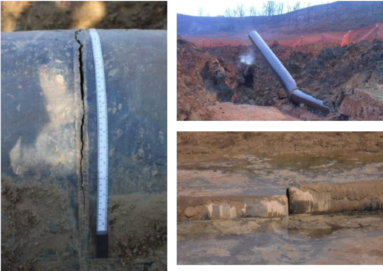
Figure 1-2 Examples of tensile failure of girth welds [1]
