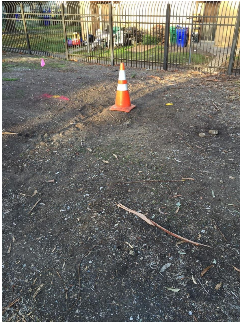
Figure 8-51 Denotes location of installed marker prior to complete backfill of pothole used for establishing baseline survey before leaving site
