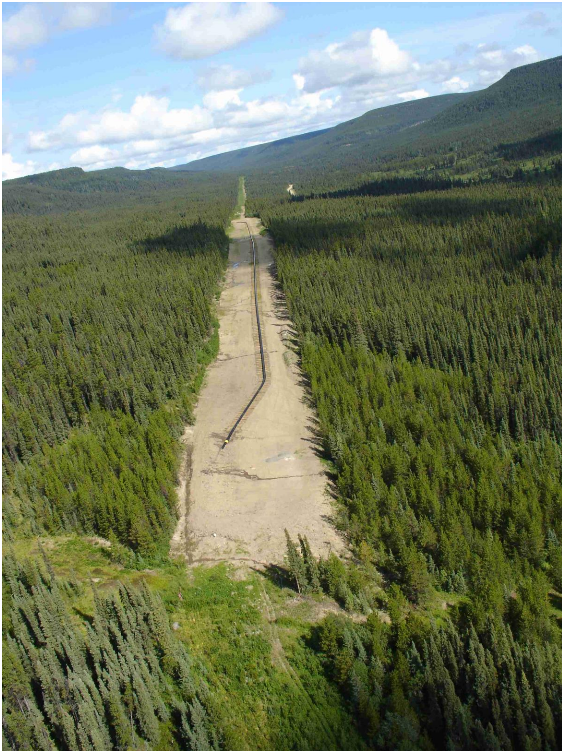
Figure 8-3 Surface pipeline segment on wooden skids for a low angle translational landslide moving from the right to left of photo (Photo by: E. McClarty, Location: Northern British Columbia, Year: 2007)
