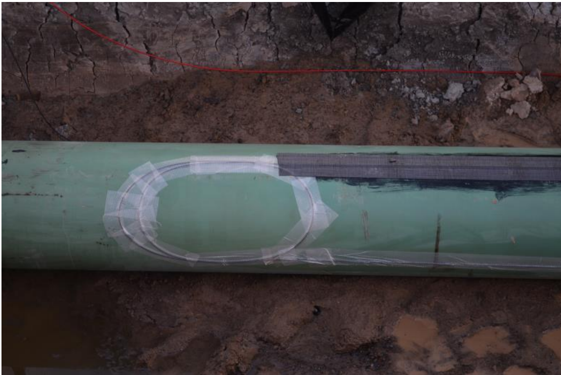
Figure 8-89 Taping a fiber optic cable top a pipe (Photo by: K. Ryan, Year: 2013)
