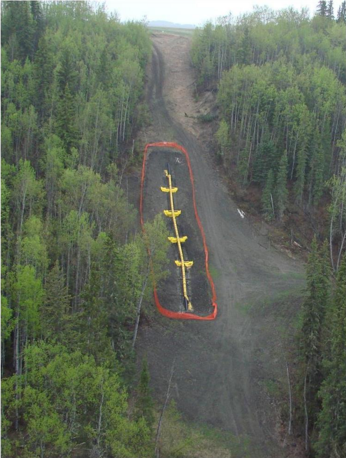
Figure 8-21 Example of stress/strain relief excavation. Trench breakers have been installed. (Photo by: E McClarty, Location: Northern British Columbia, Year: 2011)
