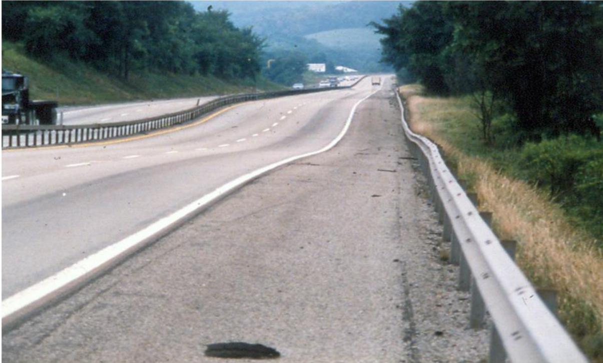
Figure 2-44 Surface subsidence trough across I-79 in Pennsylvania located above a longwall mine. (Photo by: R. Turgeon, Year: 1982)
