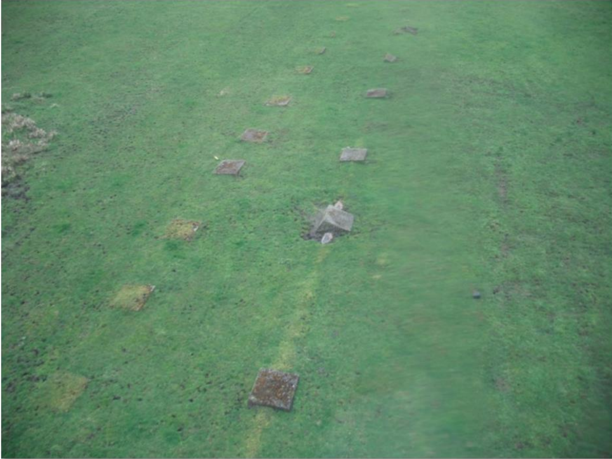
Figure 2-48 Pipeline exposure in western Washington due to drainage of organic soil which has allowed soil desiccation, subsequent loss of organic soil volume, and ground settlement (loss of ground surface elevation) around the pipeline. (Photo by: D. West, Year: 2005)
