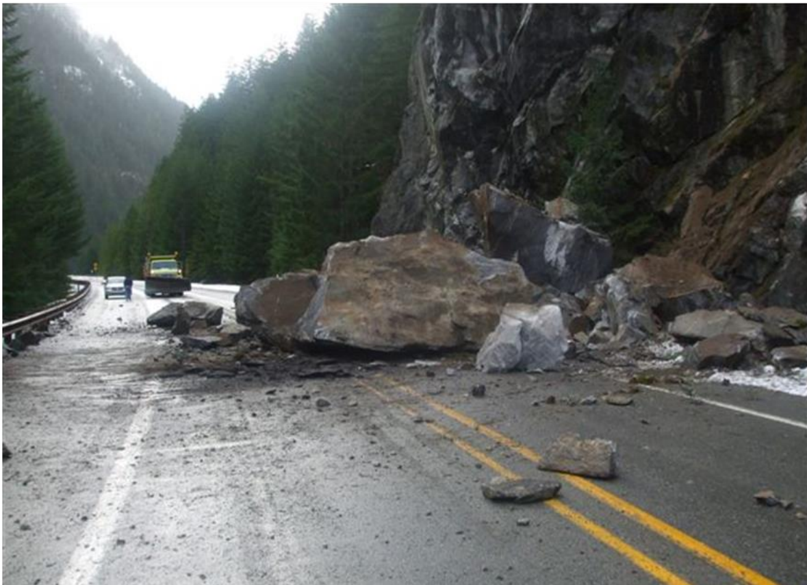
Figure 2-13 Rock fall blocks on highway SR 20 in Washington (Source: WSDOT, Year: 2011)
