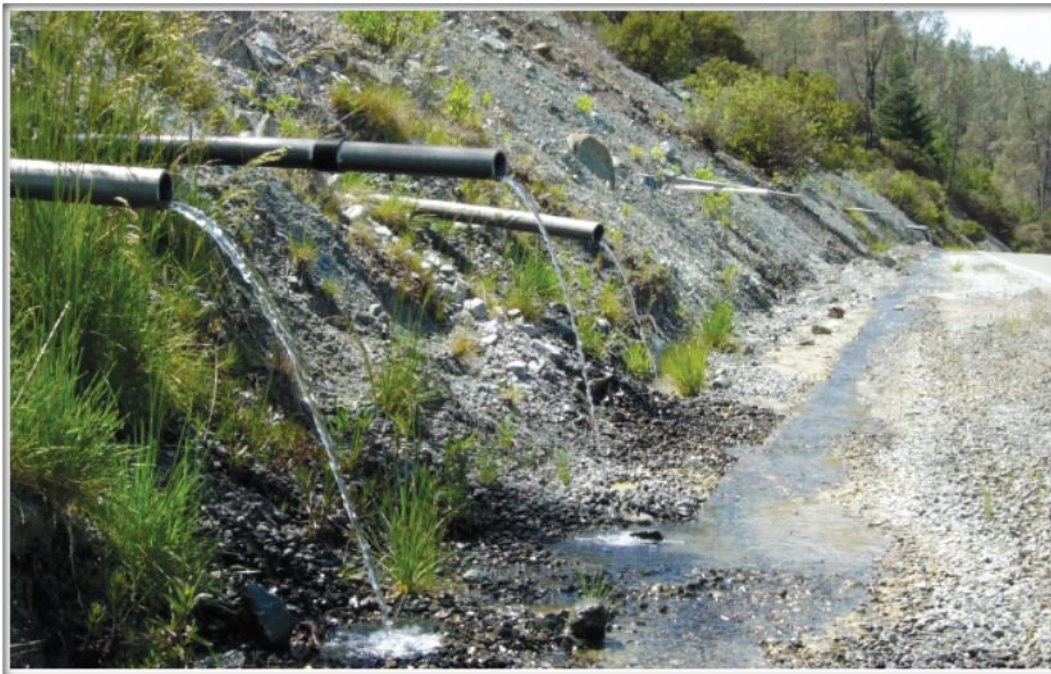
Figure 8-18 Horizontal drains on a highway cut slope [201]
