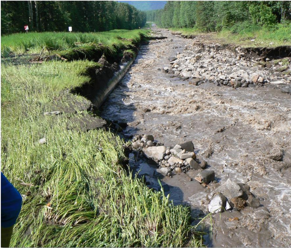
Figure 2-6 Channel avulsion on an alluvial fan triggered by an upstream log jam diverting flow down a pipeline ROW. A 36-inch mainline was partially exposed and undermined by the avulsion channel. (Photo by: D. Dewar, Year: 2011)
