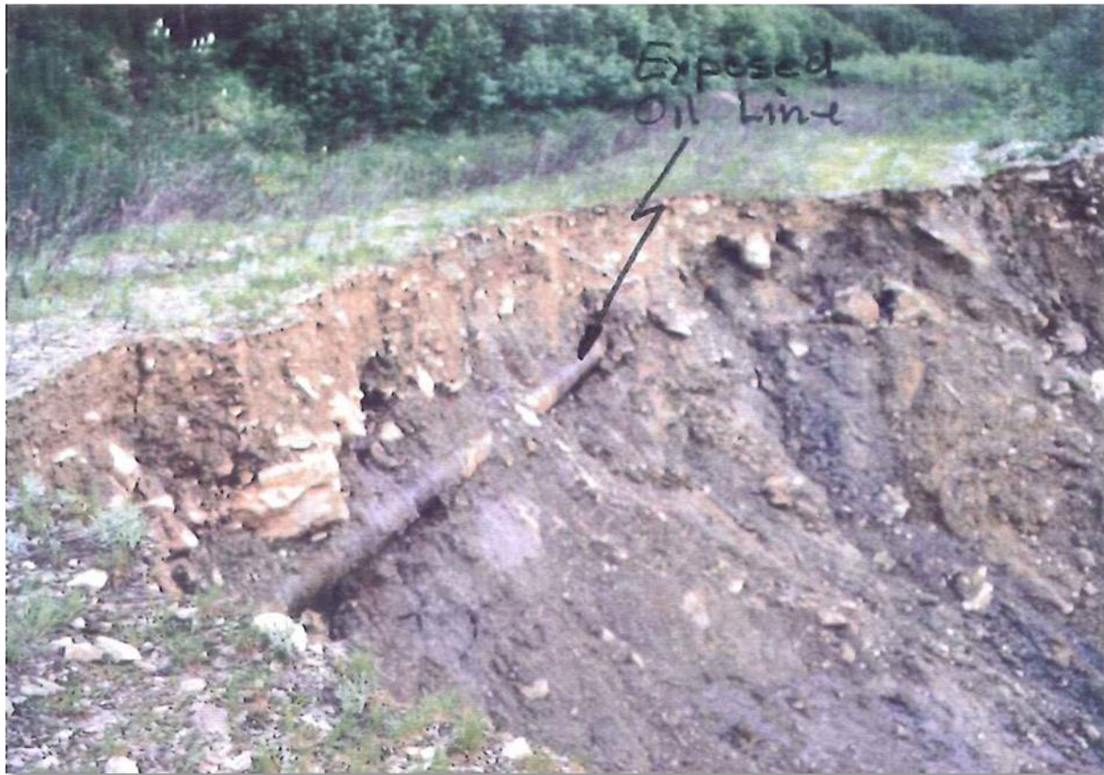
Figure 2-33 Exposed oil pipeline in the main/head scarp of a debris slide (Photo by: R. Wartlik, Location: Central British Columbia, Year: 1990)
