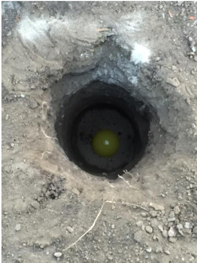
Figure 8-50 Marker ball installed at approximately 3.5 ft below ground surface, above new pipeline alignment
