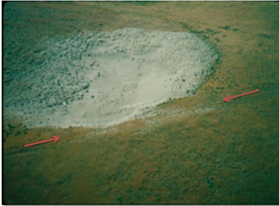
Figure 2-7 Wind erosion and deflation (lowering) of the ground surface is encroaching on a pipeline ROW (arrows) in eastern Washington. (Photo by: D. West, Year: 1996)
