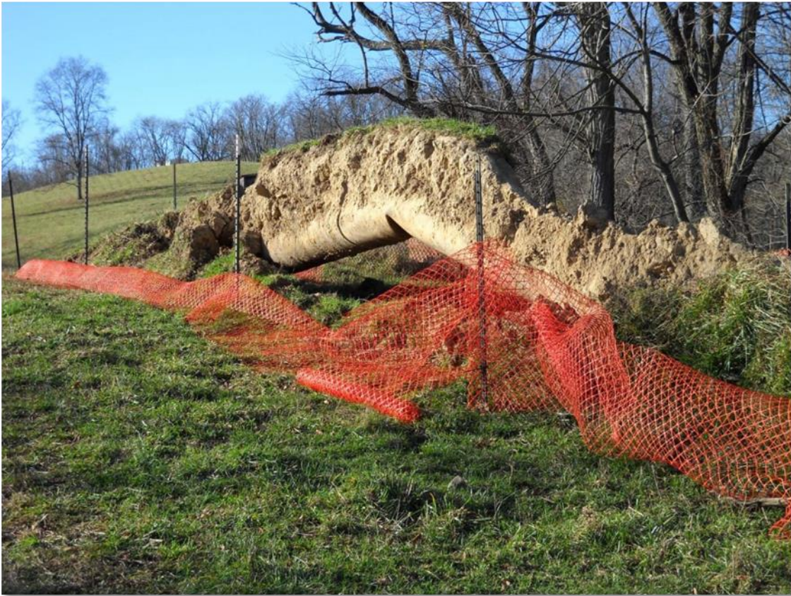
Figure 2-50 Uplifted pipe and ground breakout due to longwall mining.
