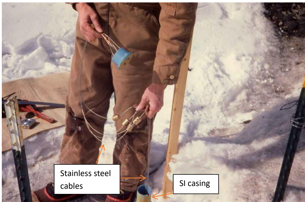
Figure 8-40 View of four extensometer cables that have been installed in PI SI casing that was being sheared-off by subsurface landslide movement. At least one of the cables was anchored below the primary, basal slip surface detected by the previous PI monitoring. (Photo by: G. Major, Year: 1987)
