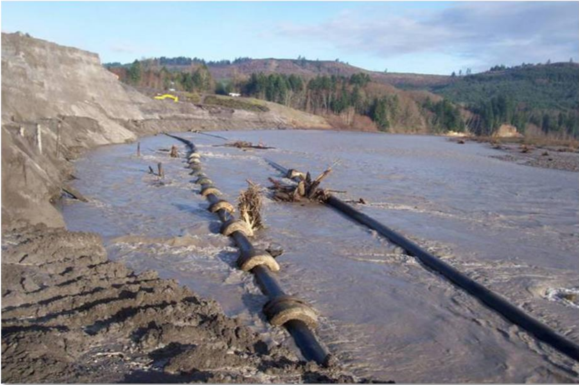
Figure 2-5 Pipeline exposure resulting from lateral channel migration and vertical erosion in western Washington. (Photo by: A. Kammereck, Year: 2007)
