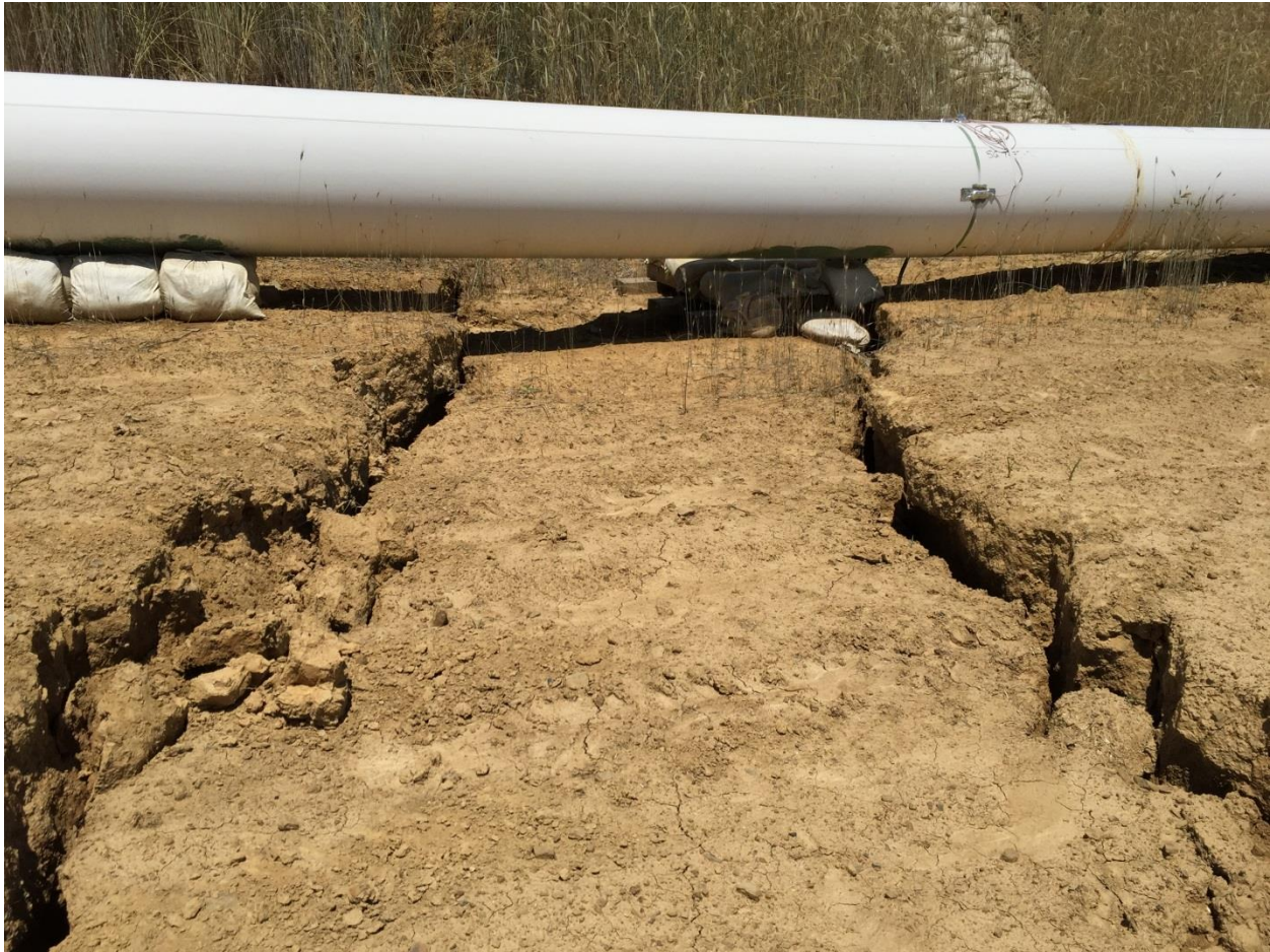
Figure 2-45 Graben at 30-inch pipeline over longwall mine in Pennsylvania
