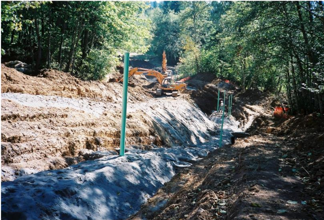
Figure 8-24 Select, clean sand backfill placed along the sides and top of a pipeline that had undergone a stress/strain relief excavation. The vertical risers are connected to trench drainage improvement plumbing. (Photo by: D. West, Year: 2002)
