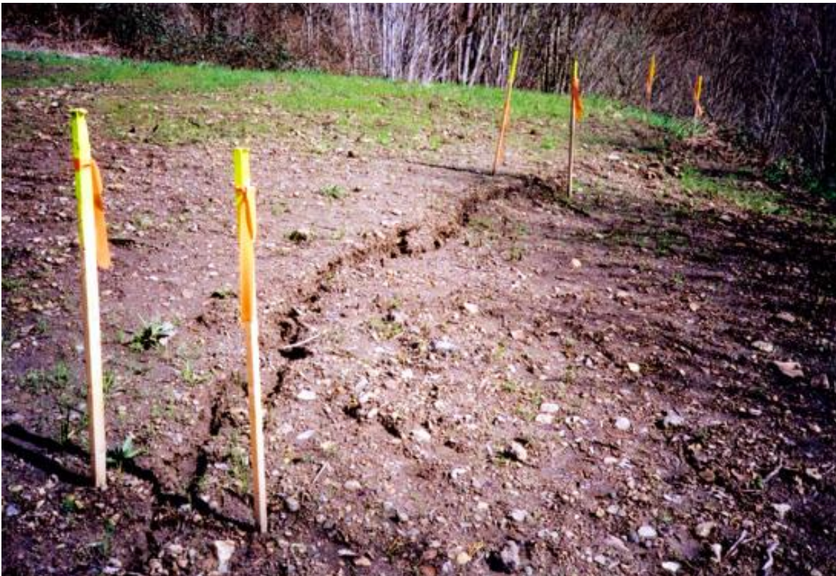
Figure 8-27 View of a landslide head scarp with survey laths placed on the upslope and downslope sides of the scarp. If each lath was visualized as a rebar, and their vertical and horizontal positions relative to each other were periodically measured, the growth of the head scarp would be documented. (Photo by: D. West, Year: 2005)
