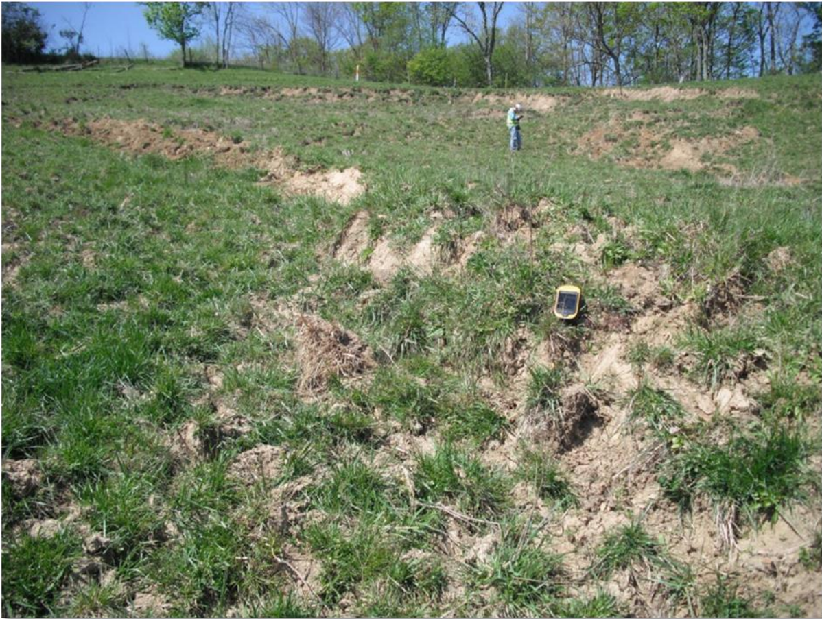
Figure 2-55 Geomorphic and geologic field mapping of an active earth flow landslide adjacent to a ROW (Photo by: D. West, Location: Ohio, Year: 2012)
