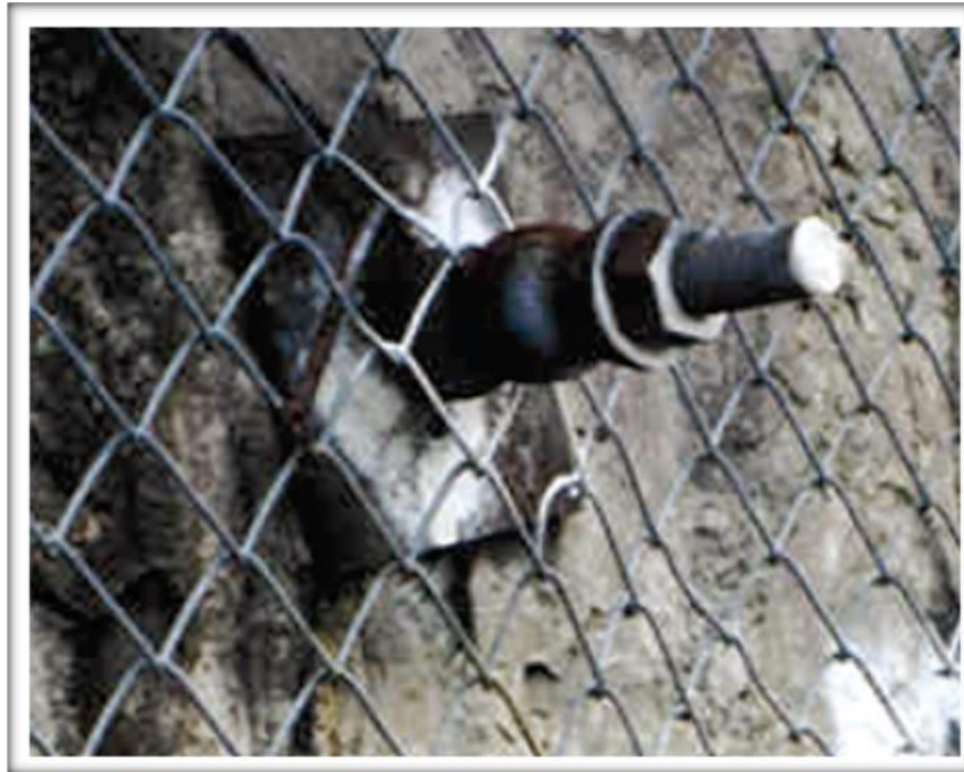
Figure 8-11 Close-up photograph of the head of a post-tensioned rock anchor on a rock face. The wire mesh provides additional containment of loose rock falling from the slope. [201]
