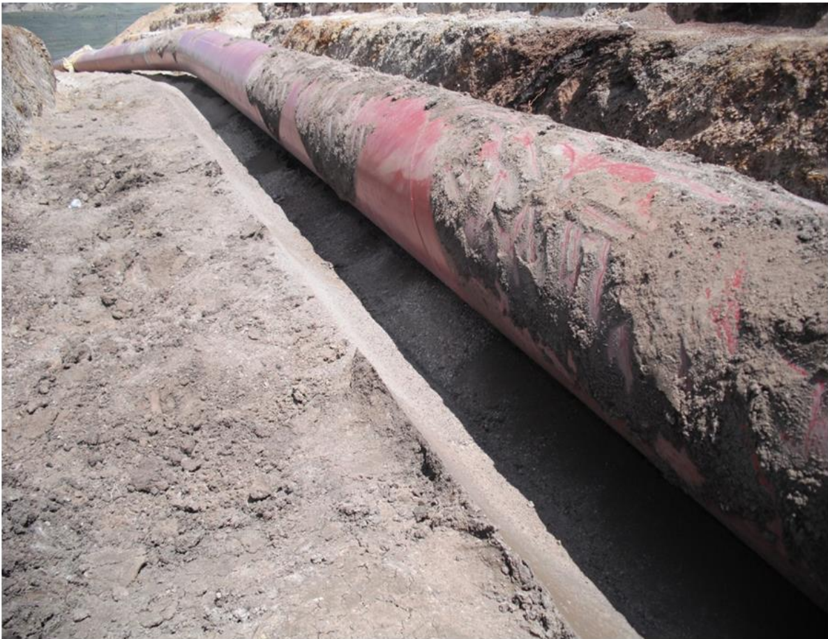
Figure 8-22 View of physical pipe lateral and vertical response in a stress/strain relief excavation for a pipeline affected by highwall landslide failures in a closely adjacent coal mine. The lateral response is about 0.25 to 0.33 times the diameter of the pipe. (Photo by: D. West, Location: The Western United States, Year: 2011)
