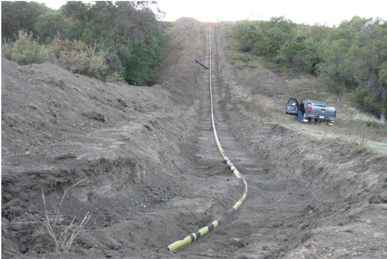
Figure 8-20 Looking upslope at stress/strain-relieved 6-inch pipeline. There is a shallow surficial slide at the top of the slope that has a toe daylighting at mid-slope. (Photo by D. Dewar, Location: Saskatchewan, Canada, Year: 2011)
