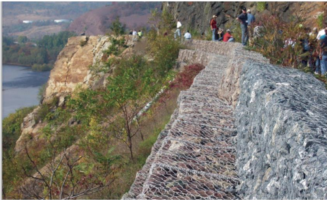
Figure 8-10 A gabion retaining wall made of individual, rock-filled gabion baskets installed on a slope above a highway embankment [201]
