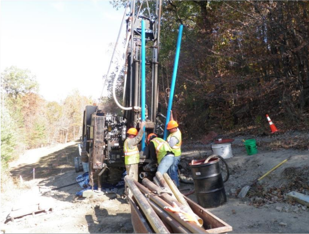
Figure 2-61 Installation of a slope inclinometer in a geotechnical exploration borehole for a Phase III landslide investigation along a pipeline ROW (Photo by: A. McKenzie-Johnson, Location: Southern Indiana, Year: 2010)
