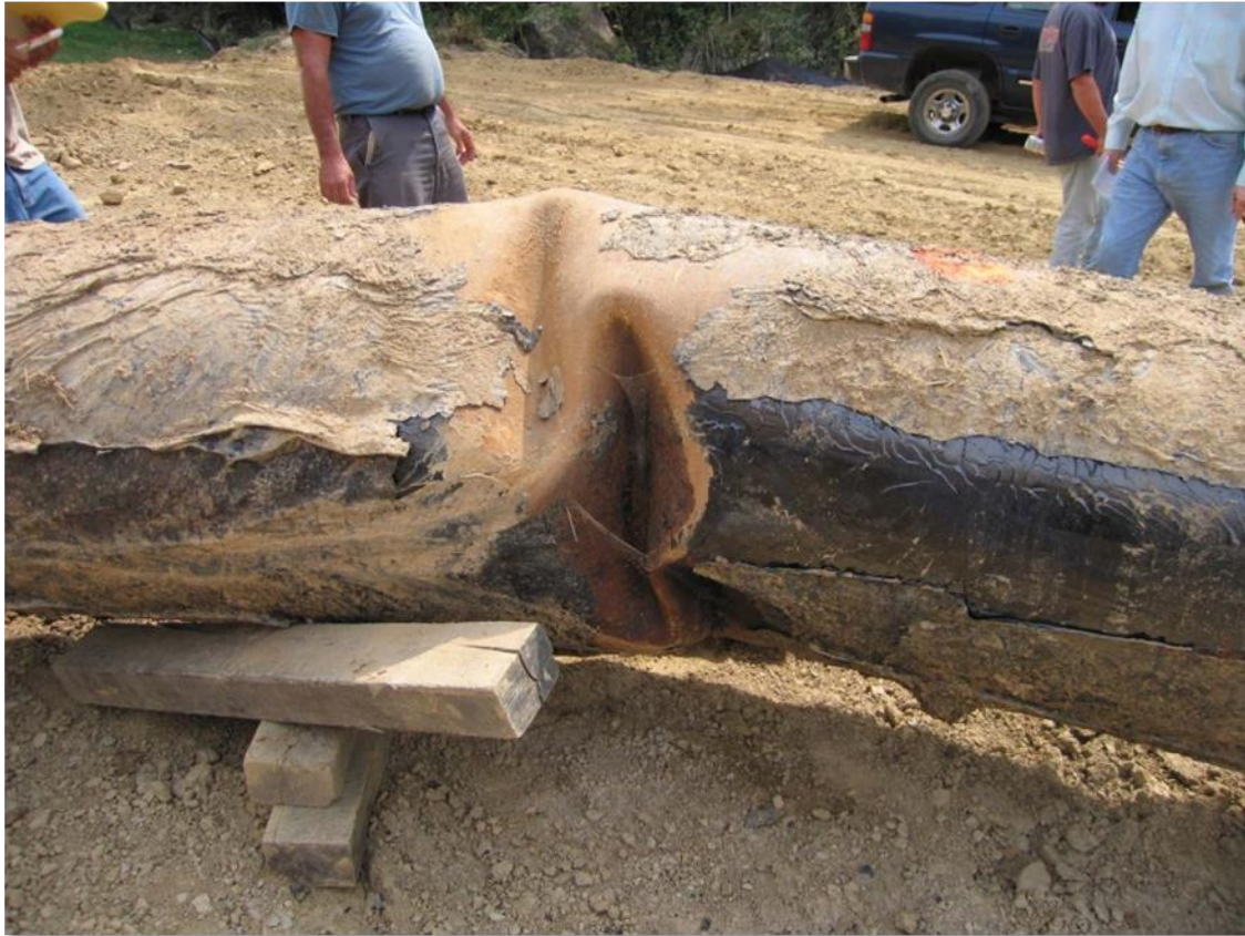
Figure 2-49 Example of pipe buckling from high axial compression resulting from longwall mining
