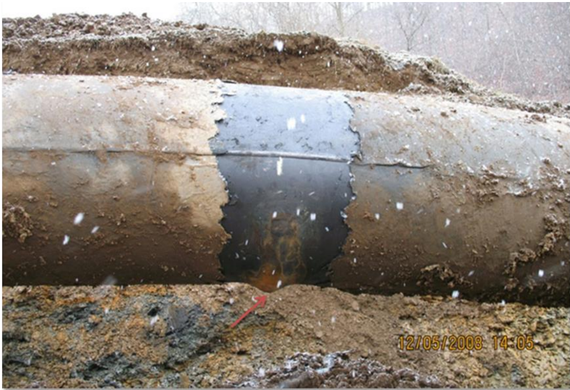
Figure 1-5 Example of pipe bulging and wrinkle formation (in-service pipeline) from axial compression due to valley closure resulting from longwall mining
