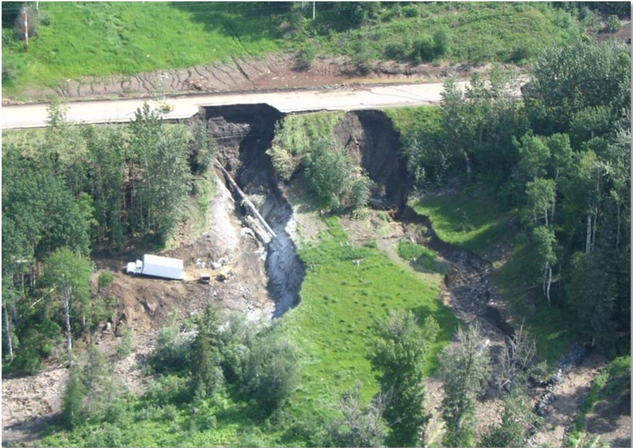
Figure 2-35 Stream diversion during high flow event that failed highway embankment exposing and free spanning 24-inch mainline. A debris flood clogged an undersized highway culvert directing water down the highway and across the pipeline ROW. A significant amount of the upstream sediment in the debris flood was derived from landslides higher in the watershed. (Photo by: D. Dewar, Year: 2011)
