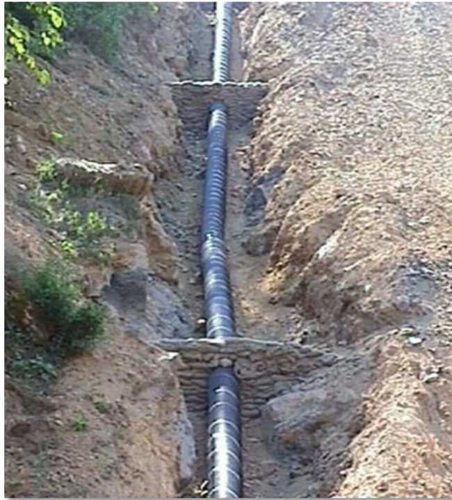
Figure 8-15 Sand bag trench breakers installed in a pipe trench to control groundwater flow in the trench. Sand bags slow the shallow groundwater as compared to clay plugs or foam breakers which are trench dams. [210]
