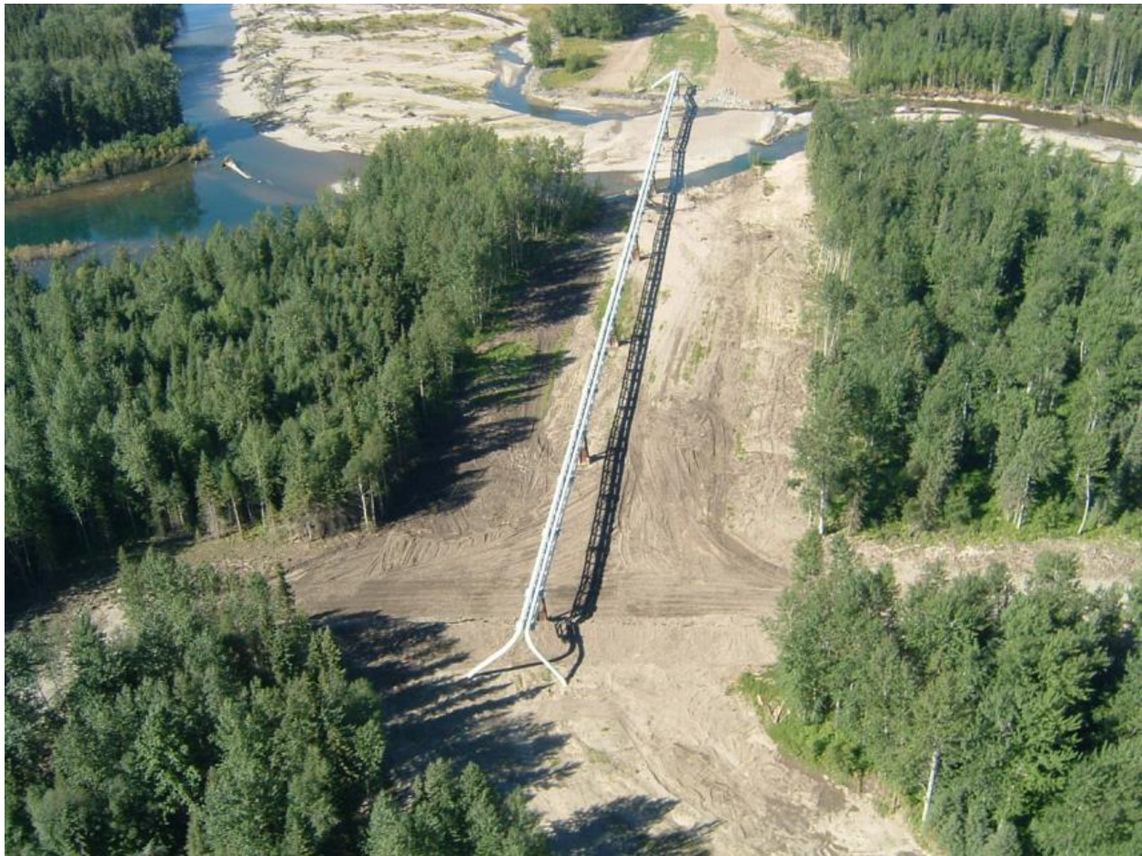
Figure 8-2 Aerial crossing constructed to reroute 30-inch and 36-inch mainline over a hydrotechnical hazard (Photo by: D. Dewar, Location: Central British Columbia, Year: 2011)
