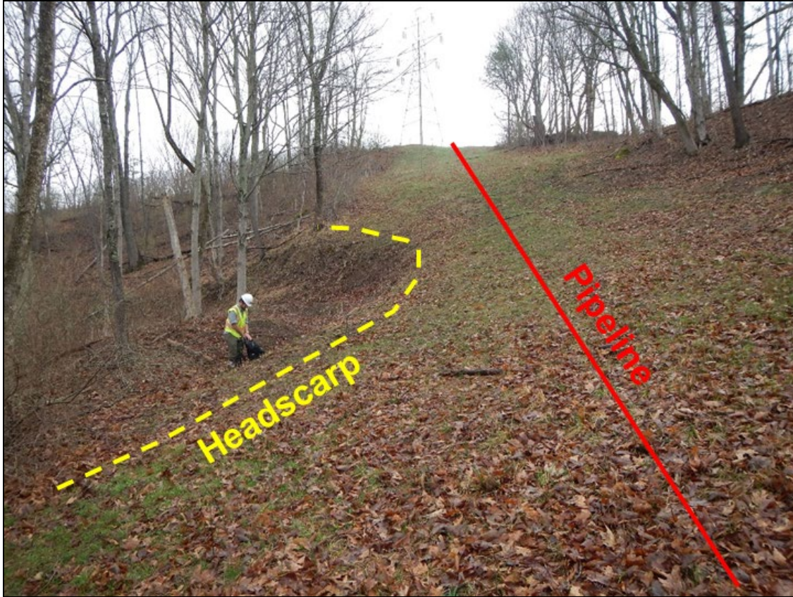
Figure 5-2. View showing a landslide headscarp (mapped during a Phase II) encroaching into the cleared ROW and approaching the pipeline centerline.
