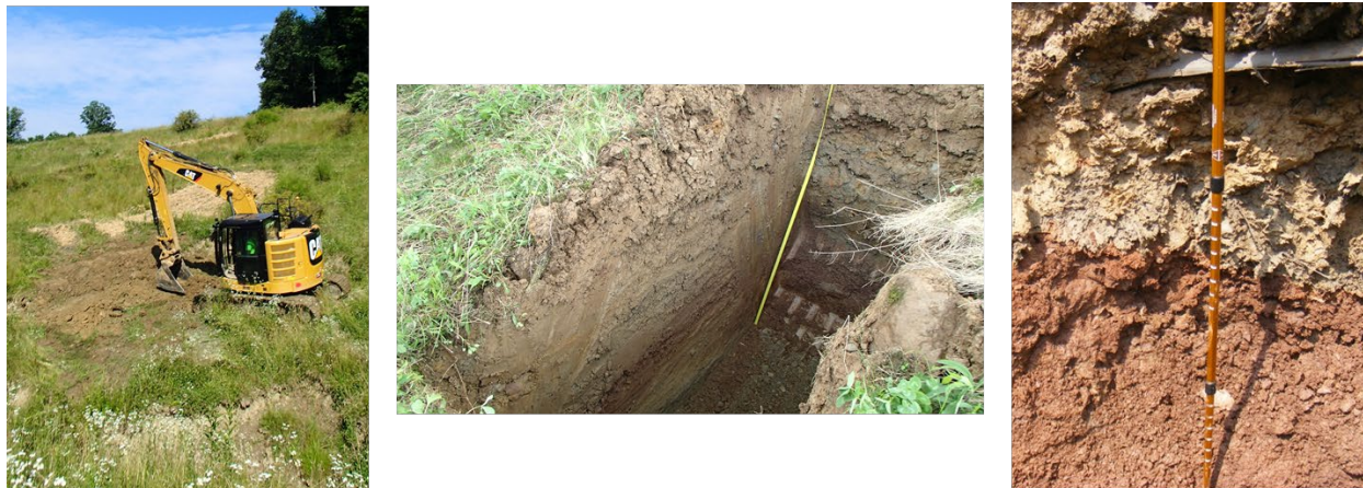
Figure 5-3. Test pit completed at a landslide site during a Phase III. Left image shows excavator prepping for excavation. Center image shows completed test pit. Right image shows the SME-interpreted subsurface boundary between landslide material (top, light brown soil) and stable material (bottom, dark red-brown soil).
