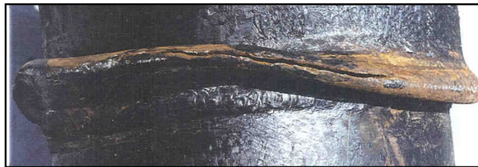
Figure 6-3. Wrinkle formation near a girth weld and the resulting cracking of pipe wall at the apex of the wrinkle
