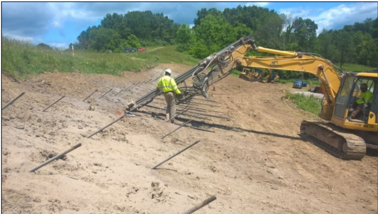
Figure 8-4. Installation of soil nails combined with site regrading to stabilize a landslide downslope of a pipeline ROW
